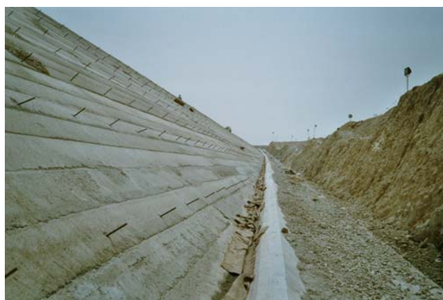
Figure 3: Optical fibres (hybrid cables) installed within a dam during construction (plinth of CFRD)
