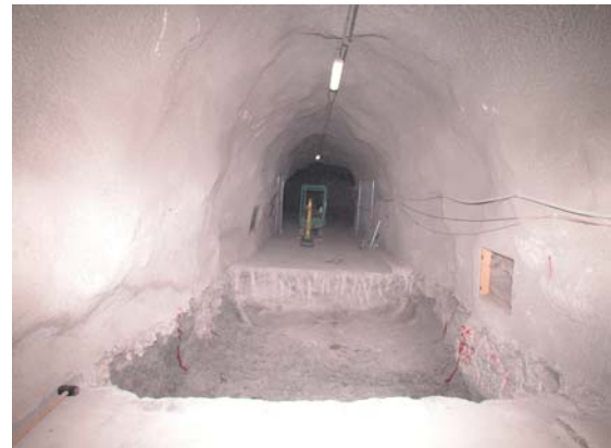
Figure 4. View of the northern entrance gallery after removing the reinforced concrete slab
