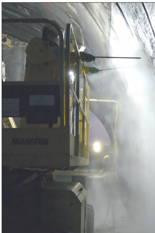
Hydrodémolition UHP jusqu'à 2500 bars / UHP hydro-demolition at pressures of up to 2500 bar.
